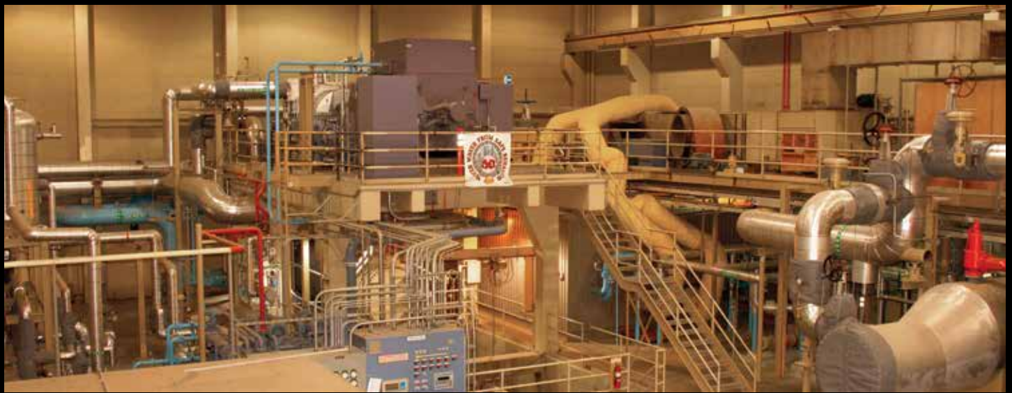
Total Energy Facility (above)
